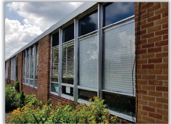
Figure CNR17.1: The Smith Government Building's single pane windows will be replaced with new heavy-duty, commercial grade, architectural, thermal windows.
