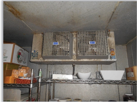
Figure E12.1: Existing Evaporator Fans
