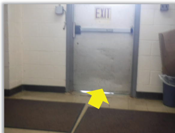
Figure E14.1: Clear daylight around the door shows a direct pathway for unwanted air leakage (Donald B. Smith Gov't Campus).
