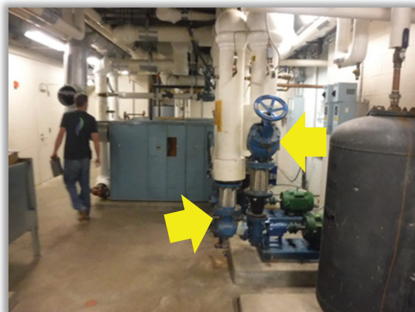
Figure E15.1: Valve & Fitting Insulation – the suction diffuser, strainer and flex fittings are not insulated which is leading to unnecessary distribution losses (New Putnam County Courthouse).
