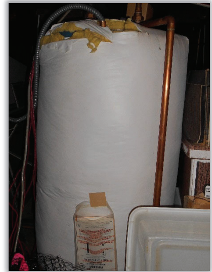
Figure CNR20.1: Existing self-contained electric domestic hot water heater tank, located in the attic storage area of the Kern Building.
