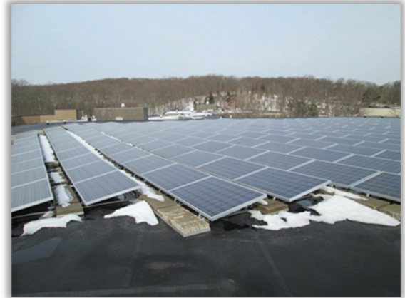
Figure E18.1: Example of a typical ballast mounted solar PV array
