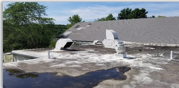
Figure E24.3: Pooling on existing flat section of roof at Golf Clubhouse
