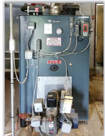
Figure E6.1: The existing boiler at the Smith Government Campus Building 3 will be upgraded with a new gas fuel train and burner.
