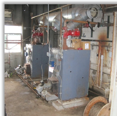
Figure E16.1: Existing boilers at the Highway Department Building 3 Dispatch
