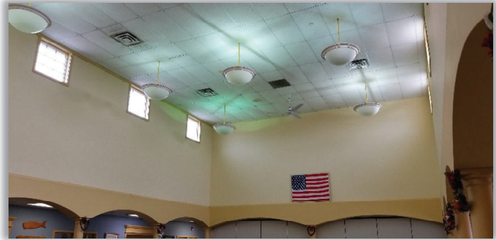
Figure E26.1: The existing supply diffusers and return grilles at the Koehler Senior Center are located close to each other and high above occupants.
