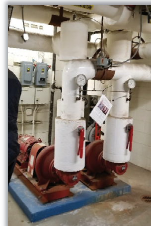
Figure E8.1: Hot water pumps
