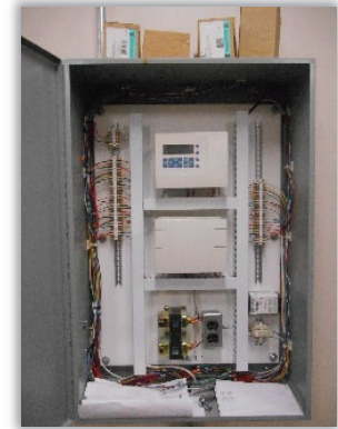
Figure E3.3: Existing Honeywell WEB-700 Controls
