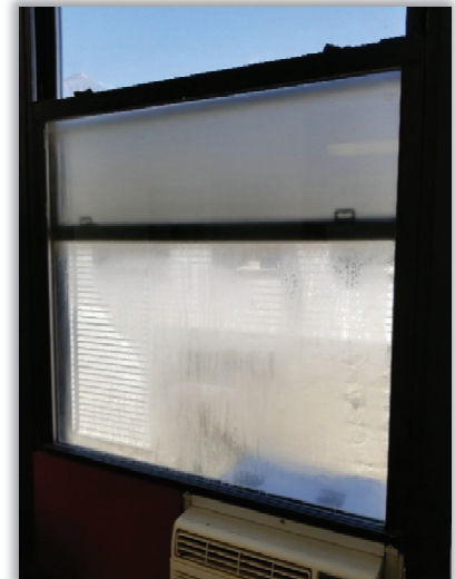
Figure E25.1 Existing double hung windows are difficult to operate and some have failed seals, causing visible clouding.
