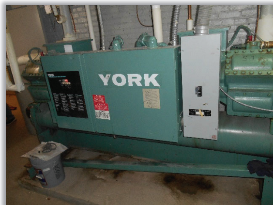
Figure E22.1: Existing chiller at the Historic 1812 Courthouse
