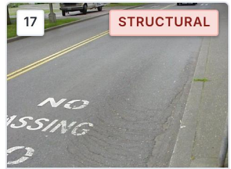
Slippage Cracking Bond failure · SF
