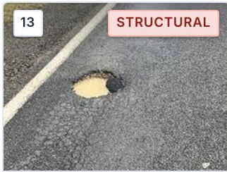
Potholes Failure · count
